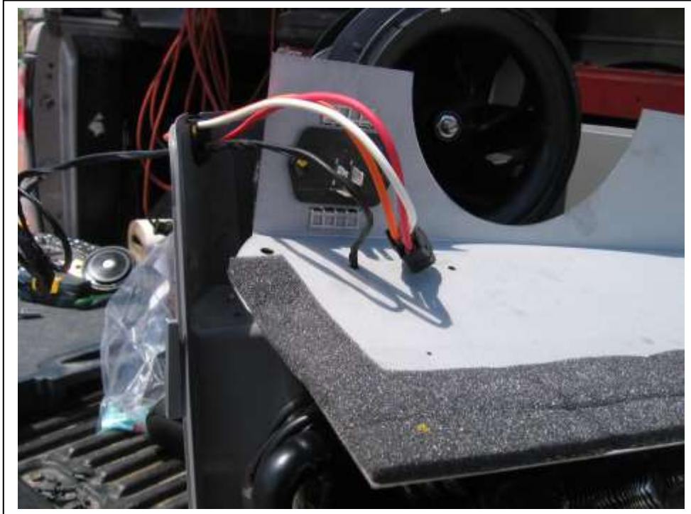
Thermostat probe coming into box. Run down through metal plate. Thermostat body gets tied up outside the evaporator box under the switch console. Find the white factory AC wire and cut and attach it to the thermostat.
